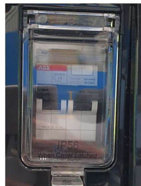
2. External Circuit Breaker
